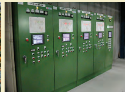
Powder and granule mixing system panel
